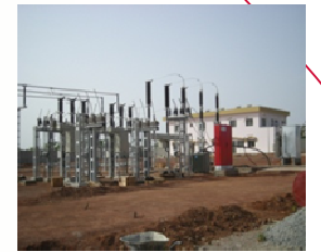
On site commissioning
