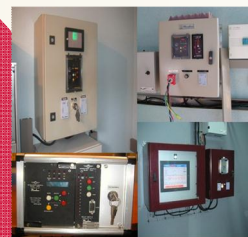
Specific relays for private power plants parallel to the EDF network.
