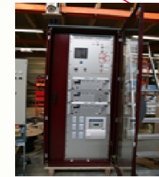
MV/HV transformers bays and line protection panels
